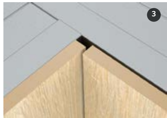
Open joint in internal corner
